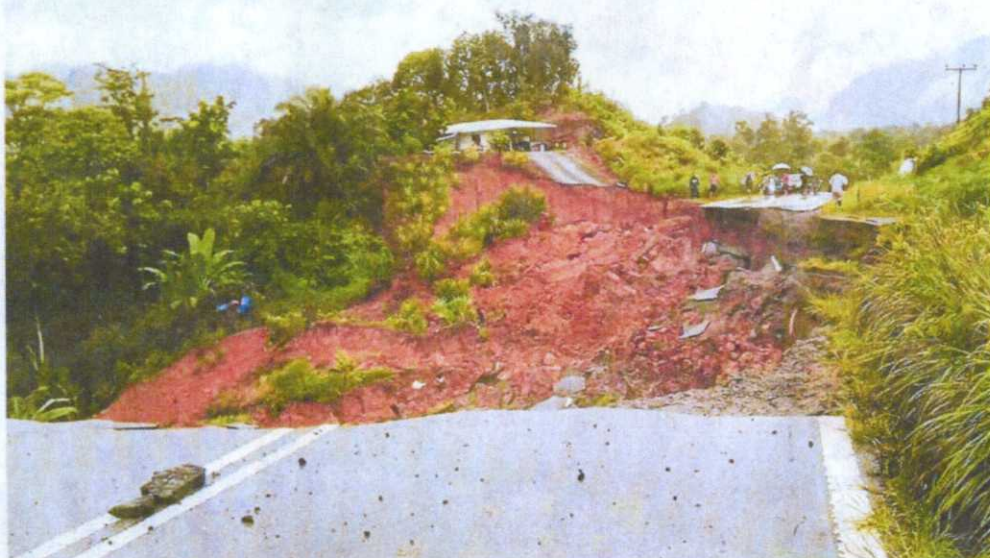
Broken Earth: A section of road at the Puncak Borneo area destroyed by heavy rain. The road, about 40km from Kuching, leads to Kampung Abang. — Photo courtesy of The Star reader
